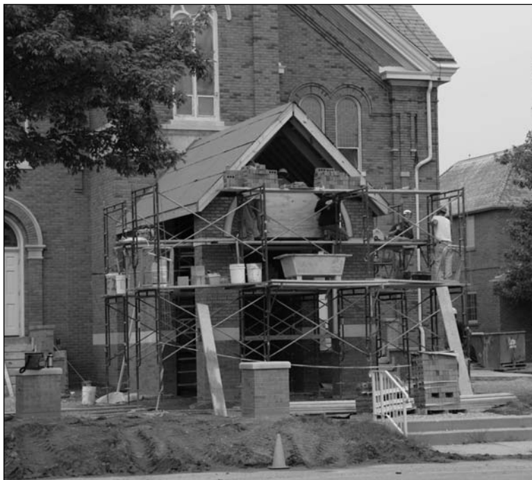
Unexpected construction on St. Michael's front steps brings the entrance back to safety.
