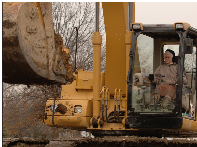
Sister Elise operates an excavator during the groundbreaking in 2006 for construction of the Pope John Paul II Center addition to Bonaventure Hall at the university.
